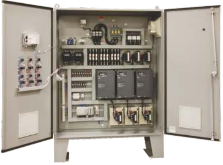
Floor mounted VFD panel for pressure boosting system
